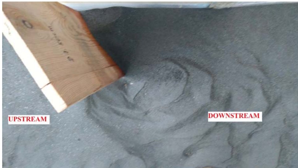
Figure 4: Extent of scour around spur dyke.
